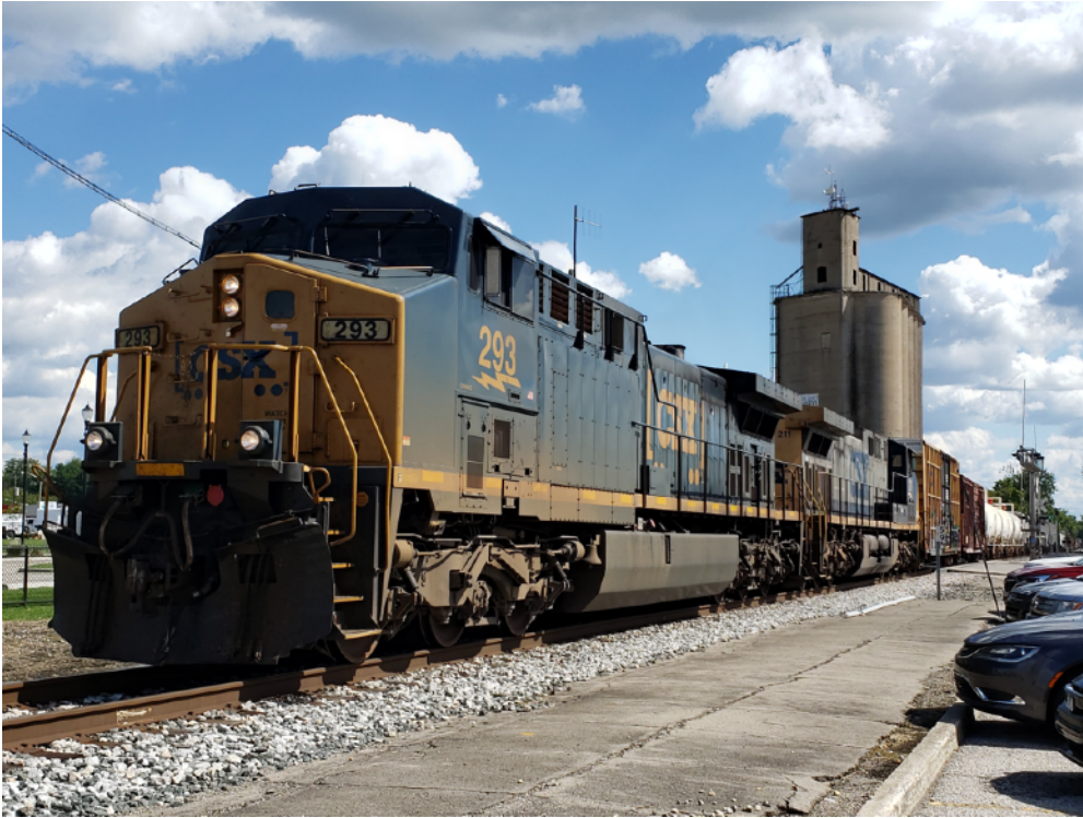
At JO Tower in Seymour, manifest Q688 (Louisville to Indianapolis) waits for the track gang and signal department to finish up PTC installation work on September 9, 2021. Once cleared, the train will continue its northbound journey over the Louisville & Indiana Railroad. Photo by Chris Dees
